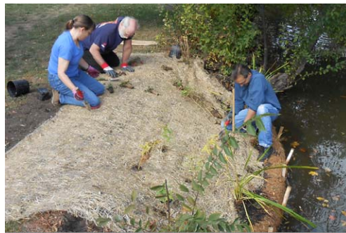
Coir logs and native vegetation was installed to stabilize eroding streambank in Northville's Historical Mill Race Village
