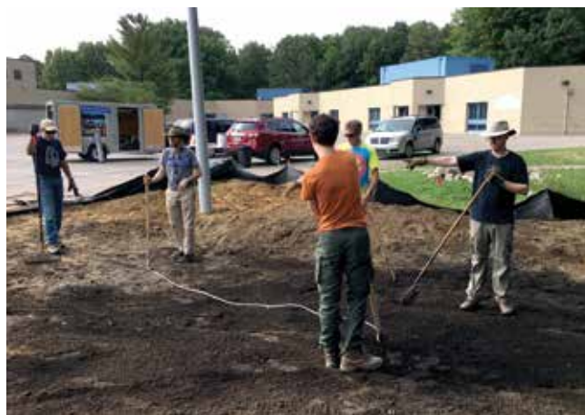
Scouts leveling the rain garden at Hulsing Elementary. Photo by Mary Weishaar-Wall
