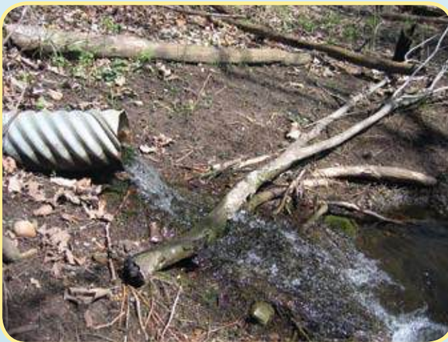
Figure 7 - Stormwater runoff entering a stream
