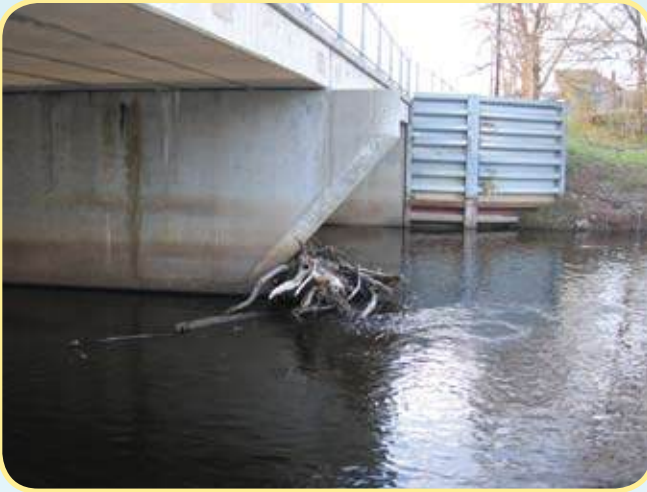
Figure 40 - Minor LWD accumulation on bridge pier
